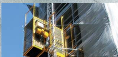
Service and goods lifts
